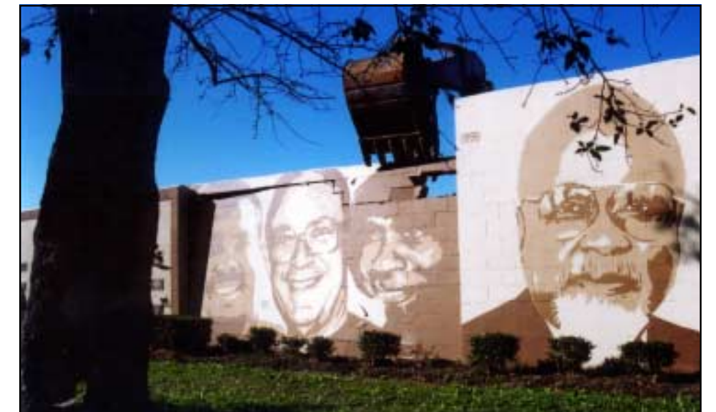
The CHA began demolition of the Wall of Fame during a ceremony on December 11, 2003.
