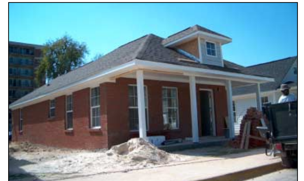
This is one of the ten cottages to be constructed as part of the HOPE VI Revitalization process. The units will house residents over the age of 50.
