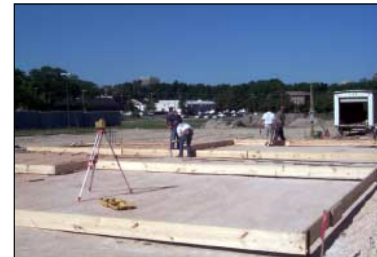
Construction has begun on five of the ten elder cottages that will be built on the Saxon Homes site. The cottages are located on the corner of Oak and Read Streets.
